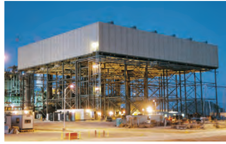
Apex, USA — ACC for 500 MW Combined Cycle Power Plant.
