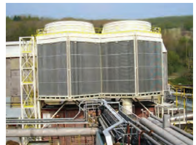
Prayon, Belgium 15 MW Cogeneration Plant
