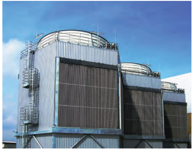
Hexacool installed in a 20MW Biomass Plant Emicheim, Germany
