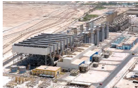
Alba, Bahrain — ACC for 800 MW Combined Cycle Power Plant. A turnkey project.
