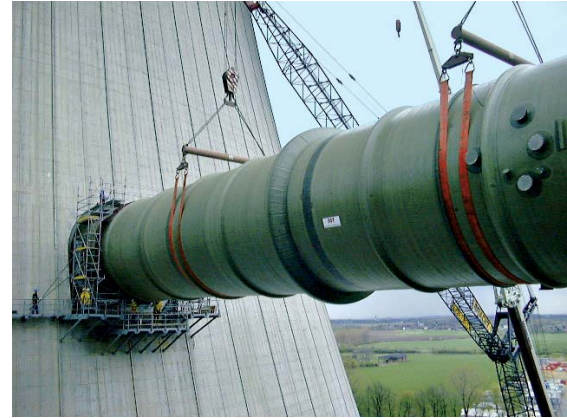
Flue gas duct entering the cooling tower of a coal-fired power station
