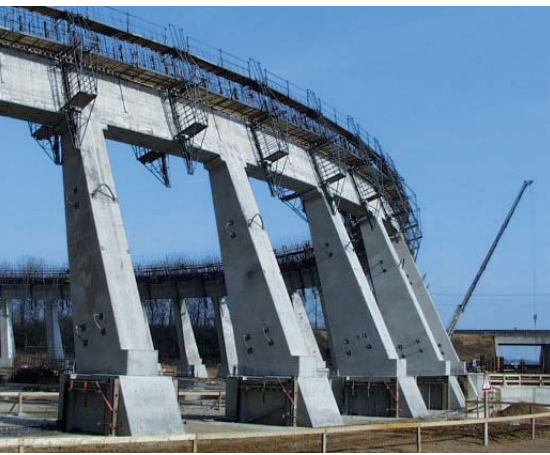
Natural draught cooling tower with meridional columns. Start of the climbing formwork.
