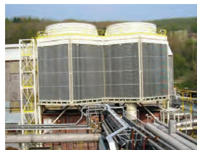
Prayon, Belgium 15 MW Cogeneration Plant
