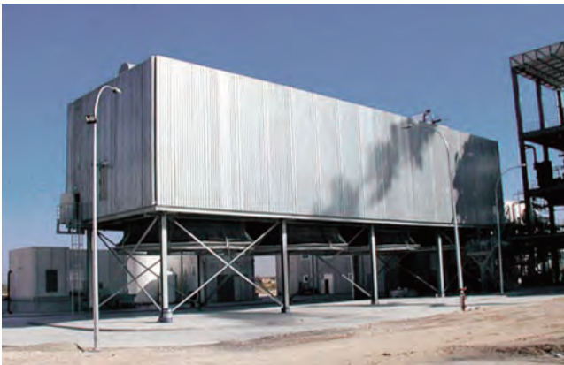
A-Frame ACC installed in a 15 MW Power Plant fueled with Dry-Waste Biomass from the Olive Oil Industry in Spain
