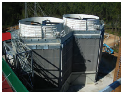
Terras de Santa Maria, Portugal 35 MW Biomass Plant
