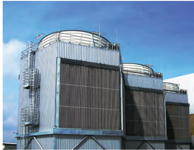
Hexacool installed in a 20MW Biomass Plant Emichheim, Germany
