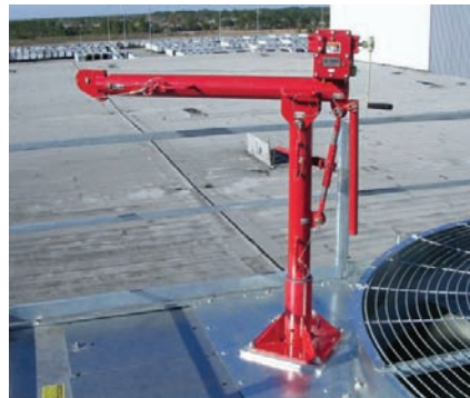
Boom reaches over fan deck railing and fan.
