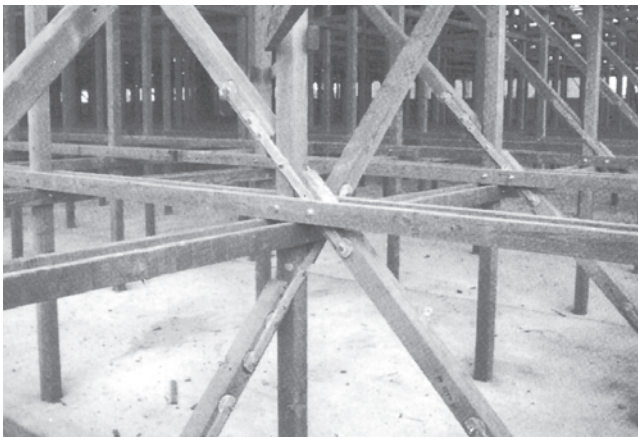
Wood structure with FRP connectors in a typical field-erected counterflow cooling tower
