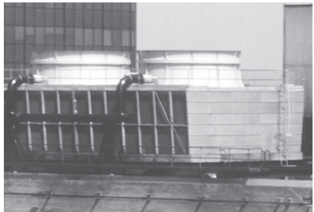
Steel structure and casing in a crossflow design.
