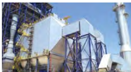
Air Pollution Control Systems
