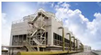
F400 Cooling Tower
