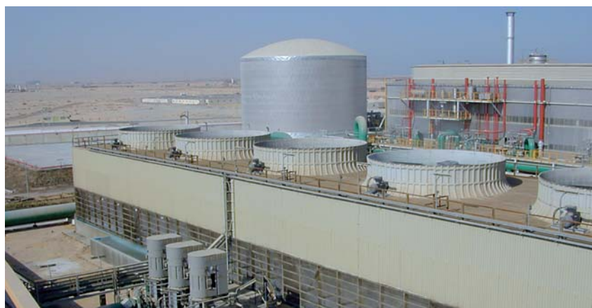
Cell cooling tower (timber construction)
