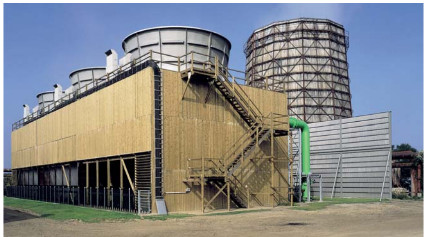
Cell cooling tower with sound attenuation wall
