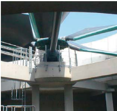
Mechanical part of an induced cell cooling tower
