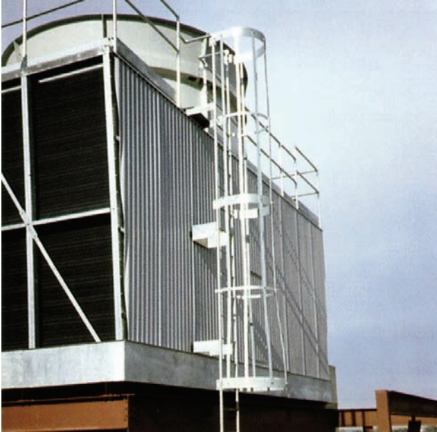
Ladder with Safety Cage
