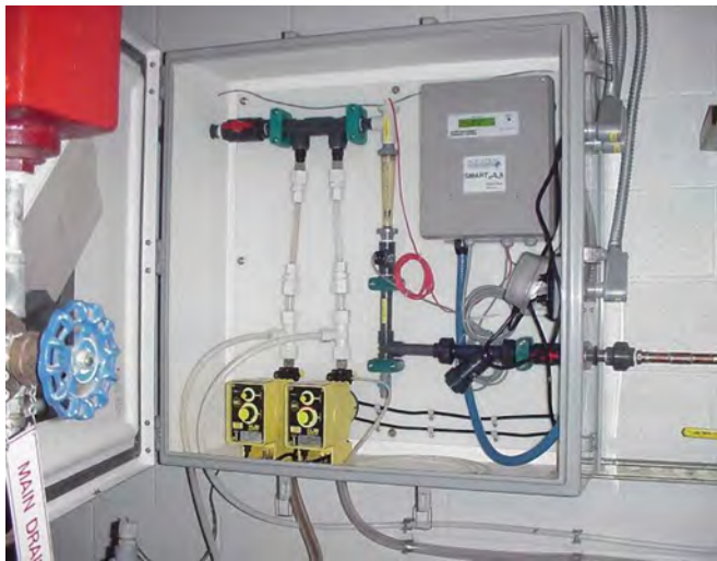
FIGURE 4 A modern packaged treatment pump and controller system is shown
