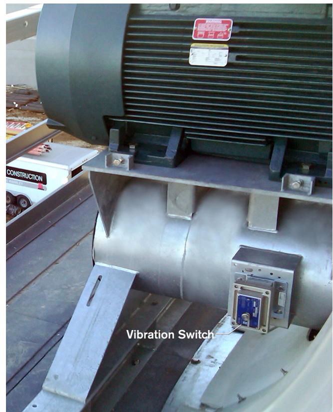
Figure 2 A mechanical vibration switch, typically mounted on the mechanical equipment support and connected to the motor starter circuit, is the simplest way to manage vibration. During an event that exceeds the setpoint, the switch can initiate an alarm and/or shut down the equipment.
