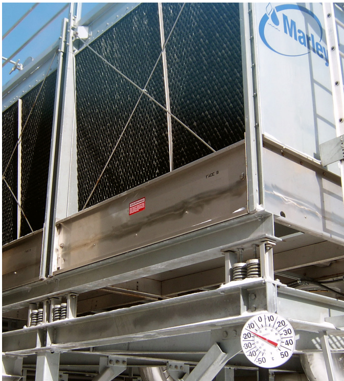
FIGURE 16 Crossflow tower in operation with integral louvers
