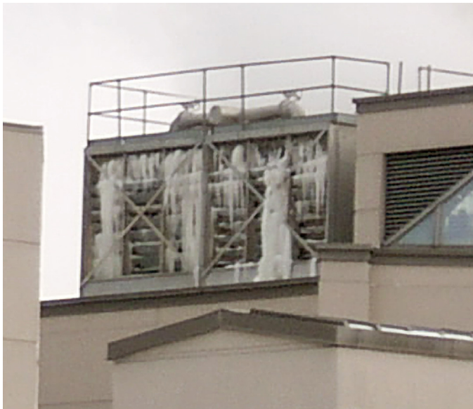
FIGURE 15 Crossflow tower in operation with blade-type louvers
