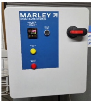
Figure 25: Panel Enclosure Photo
