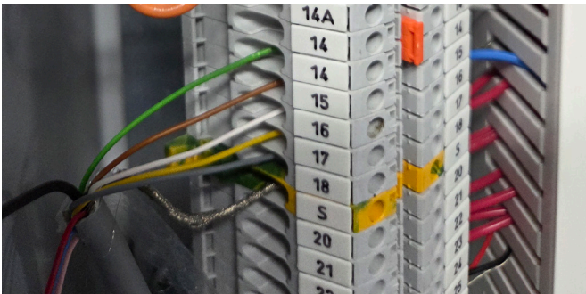
Figure 7: Sensor Terminal Block Wiring
