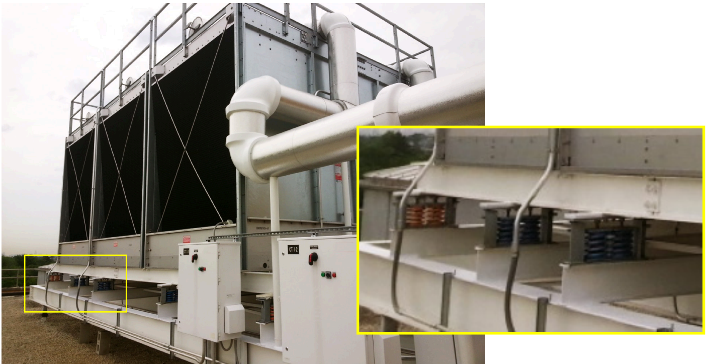
Vibration Spring Isolators located below the supporting steel on a multicell cooling tower
