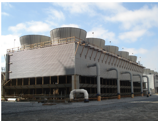
Field-erected (FEP) cooling tower – induced-draft counterflow cooling tower
