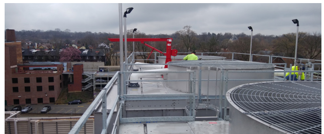
Nine cooling towers were replaced during two phases scheduled a year apart.
