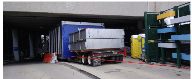
The installation required the cooling towers to be transported by truck under a multi-story parking garage.
