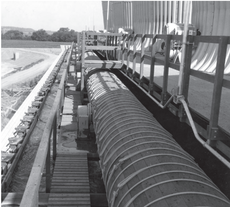
Figure 130 — Ladders, guardrails, and access-ways on a crossflow tower. Note wood stave pipe header (no longer current).
