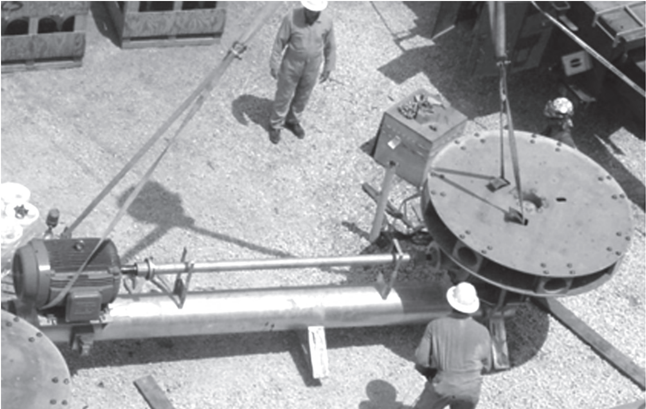
Figure 69 — Mechanical equipment mounted on torque tube, before installation of fan blades. Note retaining guards for driveshaft.
