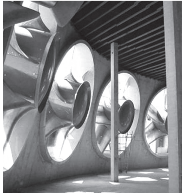
Figure 7 — Inside of a fan-assisted natural draft tower.
