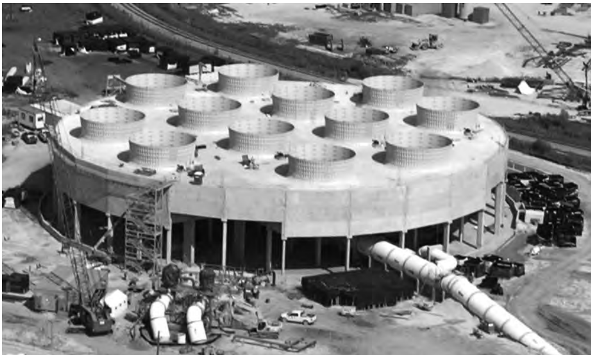
FIGURE 5 Multifan common plenum cooling tower
