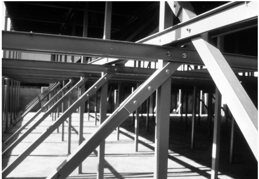
Marley pultruded FRP structure
