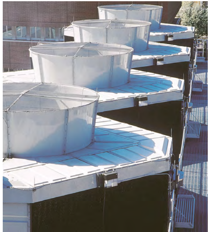
A modern cooling tower features construction materials of fiberglass, stainless steel and PVC
