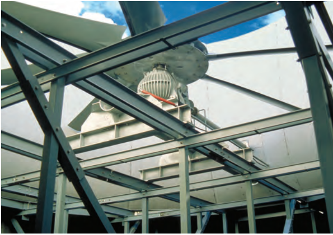
Pultruded FRP in a typical field-erected counterflow cooling tower
