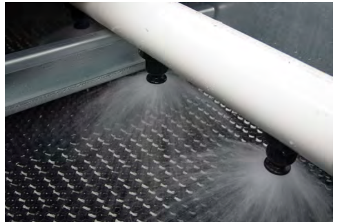
PVC distribution system piping with polypropylene nozzles
