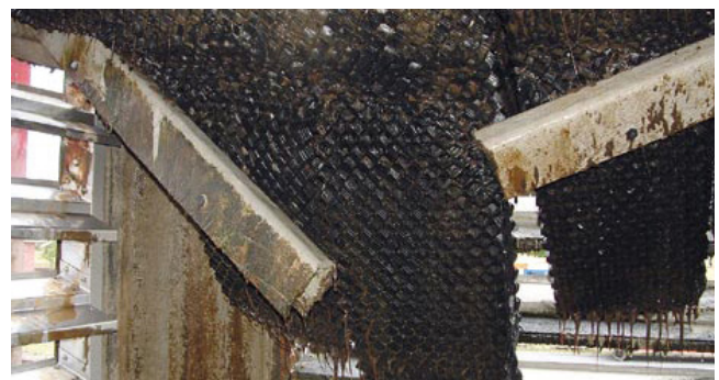
Structural Collapse Caused By Biofouling
