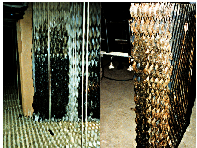
Biofouling of Counterflow Film Fill
