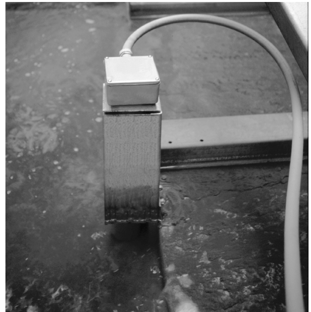
Electrode Probe installed in a Marley NC ® cooling tower
