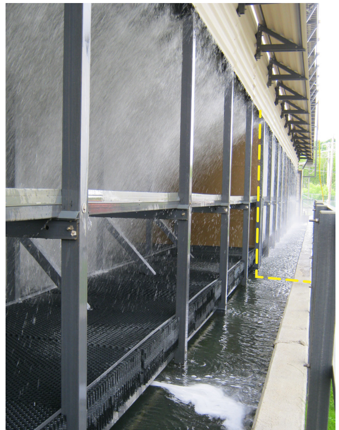
Counterflow Cooling Tower – Fan is on in near cell, but off in further cells. Note splash-out and small cloud of mist (aspiration), both common with fans off.
