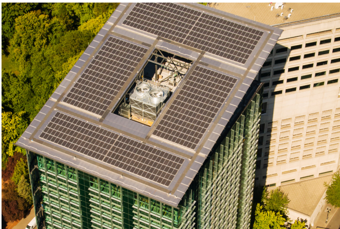
Evaporative cooling towers installed atop the LEED Platinum certified Edith Green-Wendell Wyatt Federal Building in Portland, OR
