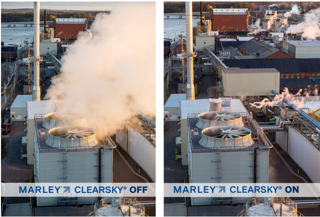
Field-erected cooling tower using plume abatement technology.
